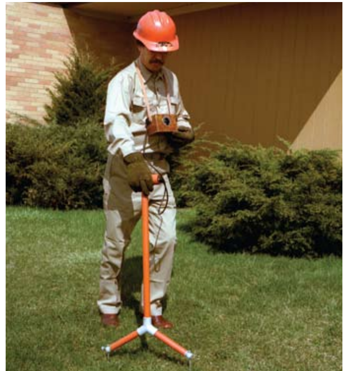
Locating the fault.
